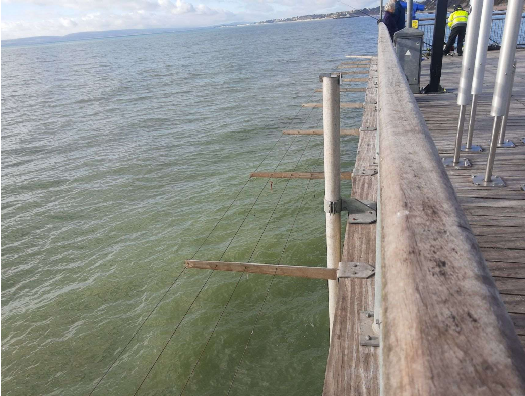
Figure 6: Boscombe Pier, anti fall/jump fence. The wires are spaced 200 mm apart, start at 380 mm from the pier edge and the outriggers are 1200 mm long. The distance from the handrail centre to the pier edge is 310 mm.
