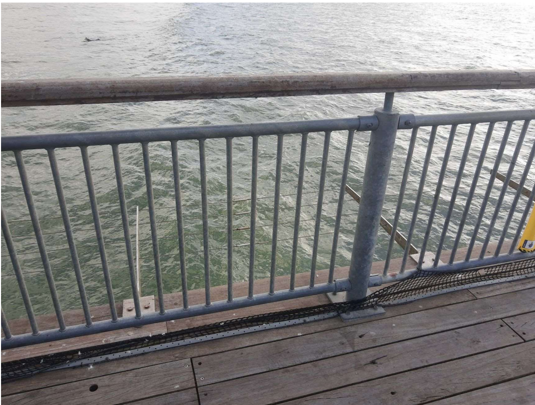
Figure 5: Boscombe Pier, handrail and anti fall/jump wires. Spacing of the handrail uprights is 100 mm, each field has a span of 2400 mm. The horizontal bars have a diameter of 50.8 mm and the uprights are 10 mm. The upright mounting the handrail to the pier has a diameter of 103 mm.
